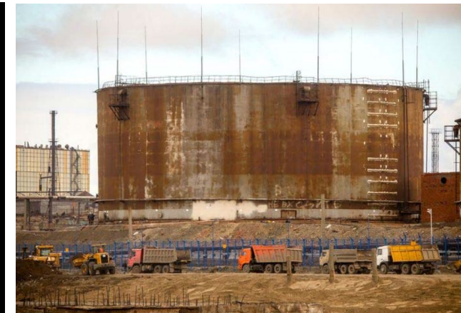
Crumbling industrial legacies Thaw-damaged diesel tank, Norilsk power plant, causing the largest Arctic diesel spill so far (~22,000 t diesel) (Source: AFP)
